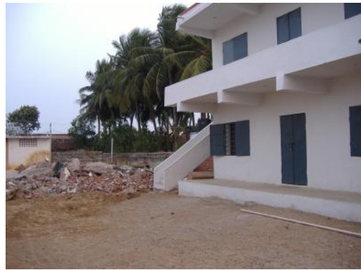
The new Government building and, to the left, the rubble of the old classroom where now a splendid two storey building is going up.
